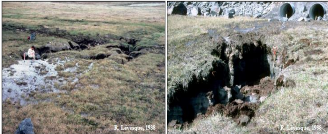
Figure 13 : Thermo-erosion that developed at the culvert outlets after the airport access road construction in 1988 in Salluit (Allard et al. 2010).
