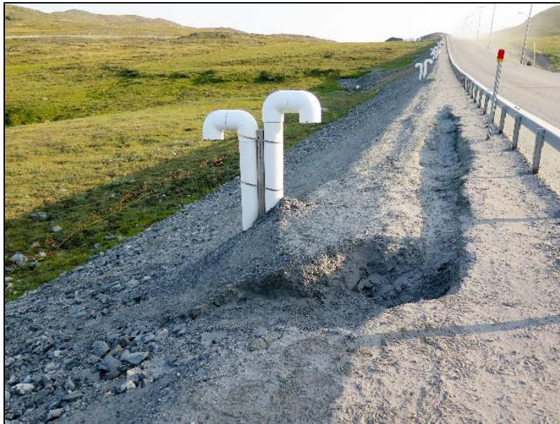
Figure 17 : Erosion scars observed on one of the embankment shoulder
