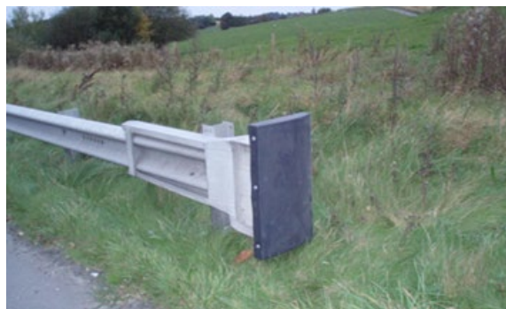
Deformable safety barrier end te
