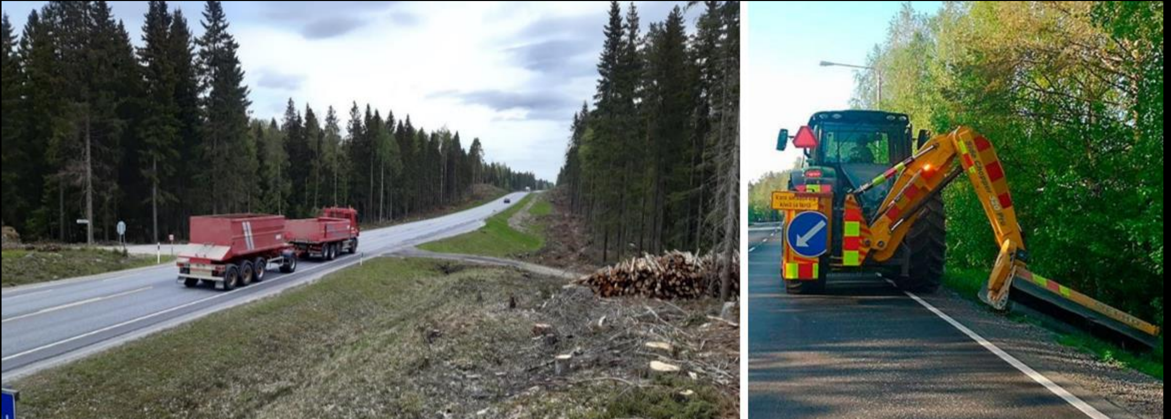
Figure 8 - On Highway 10, forest has been cleared within 30 m of the centre line of the road towards the forest in the deer warning area and the branch height has been increased by 2.5 m.
